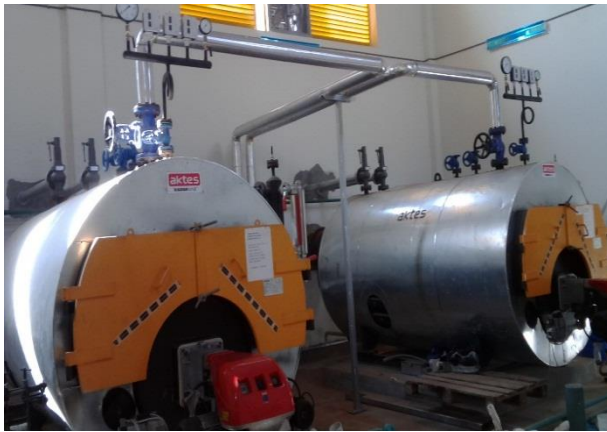
2TPH Steam Boiler, Towa
