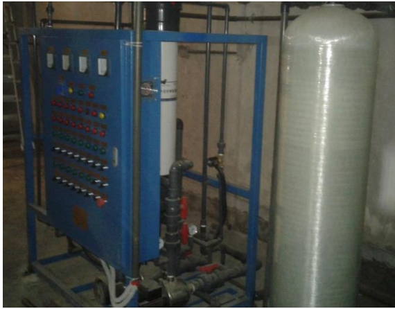
UF System (WWTP), BTI Tower
