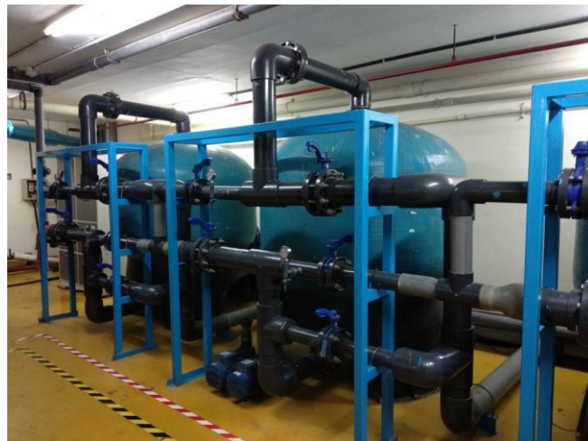
Water Treatment Plant, Saiham Tower
