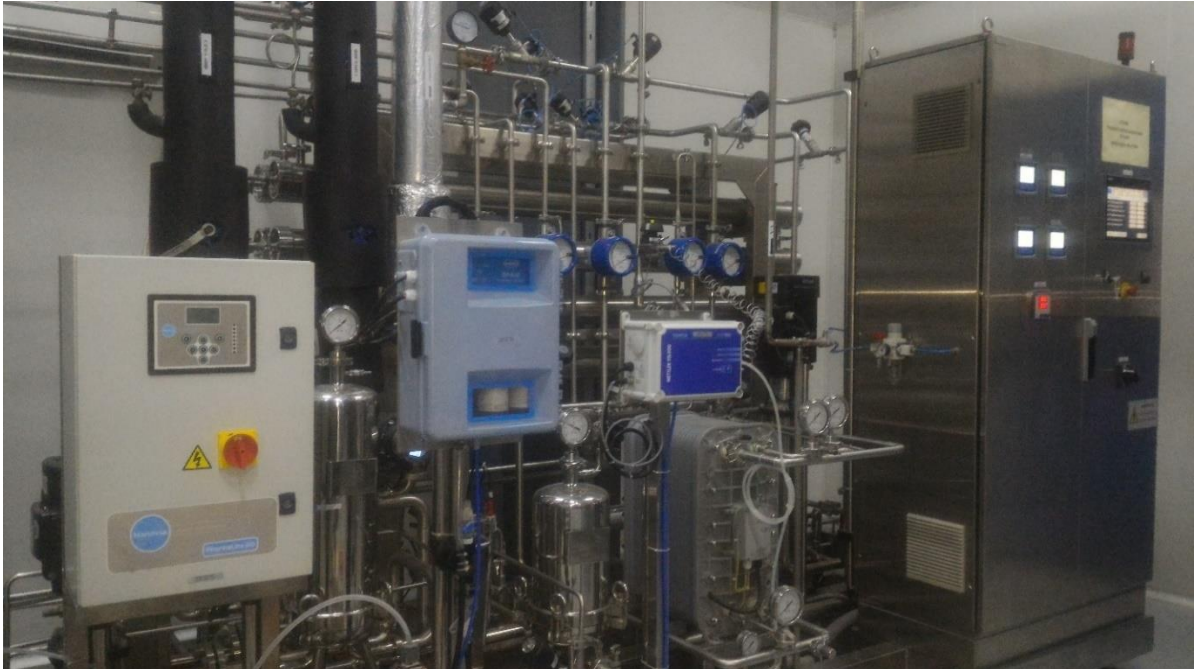
Purified Water distribution system, ACI Healthcare Ltd.
