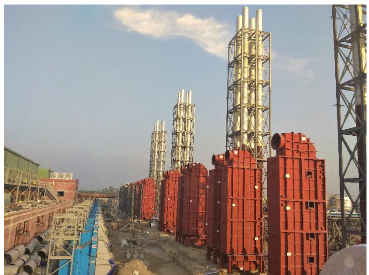
Exhaust Gas Boiler, Confidence Power Rangpur Ltd.
