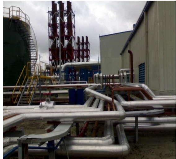
Meghnaghat 100 MW HFO Power Plant
