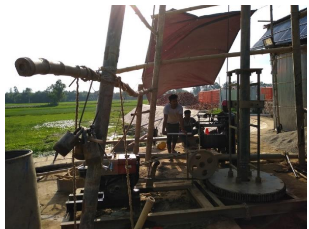
100 CMH Deep Tube well, CPRL
