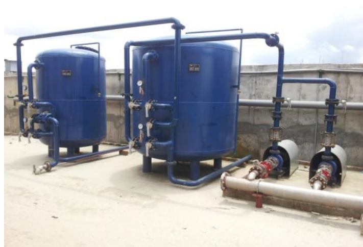
IL Bangla Ltd., Pre-treatment System
