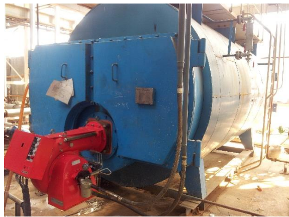
Oil Fired Steam Boiler, Greens
