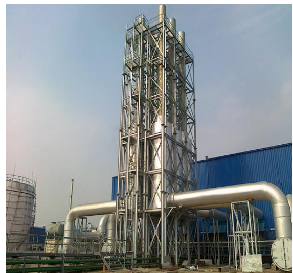
CPCL 50MW HFO Power Plant
