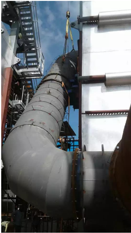
EGB Duct Boiler, OPRL
