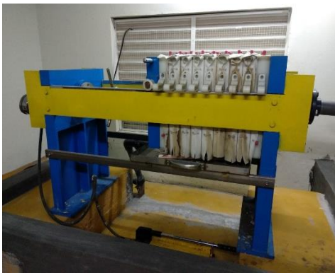
Filter Press, Saiham Tower
