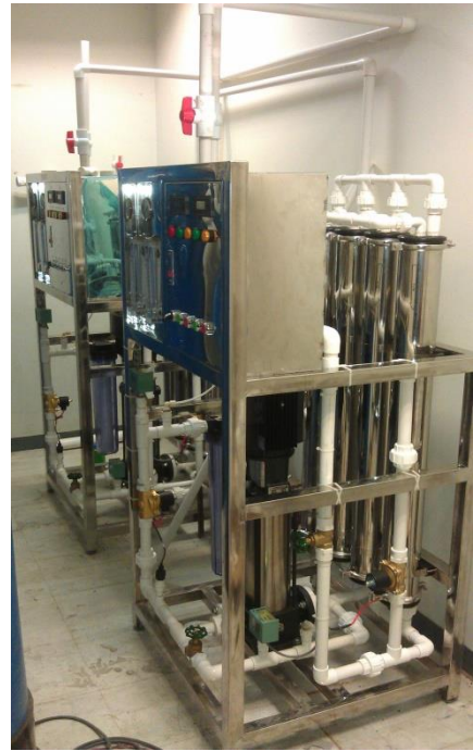
WTP(Dialysis), Square Hospital
