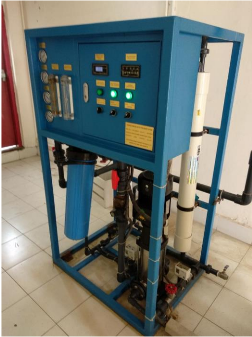
Drinking water system, Saiham Tower
