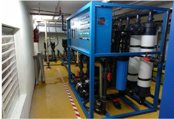
UF filter (WWTP), Saiham Tower
