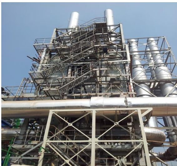
BPPL 53.3MW HFO Power Plant
