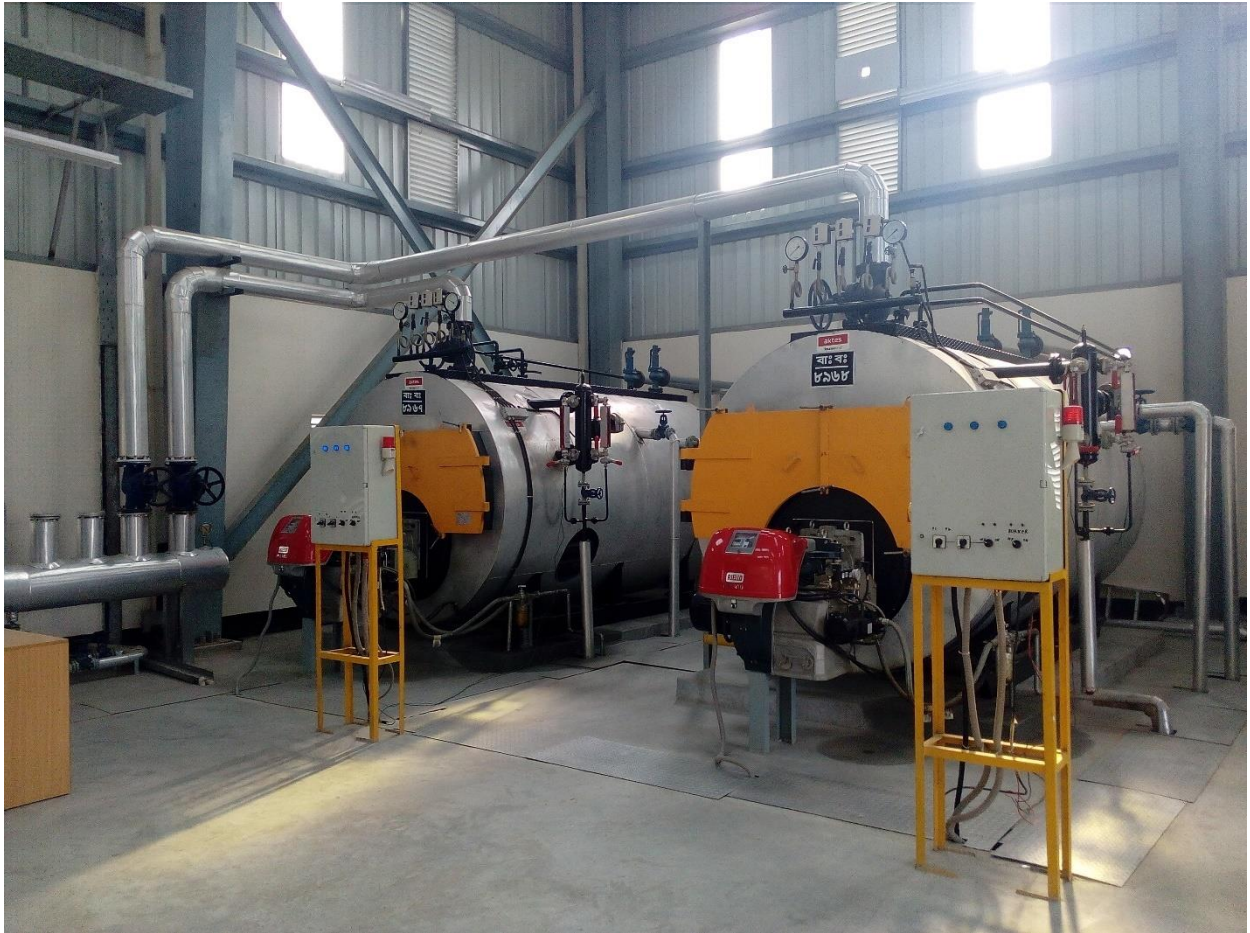
2 Set 4 TPH Aktes Steam Boiler, ACI Healthcare Ltd.
