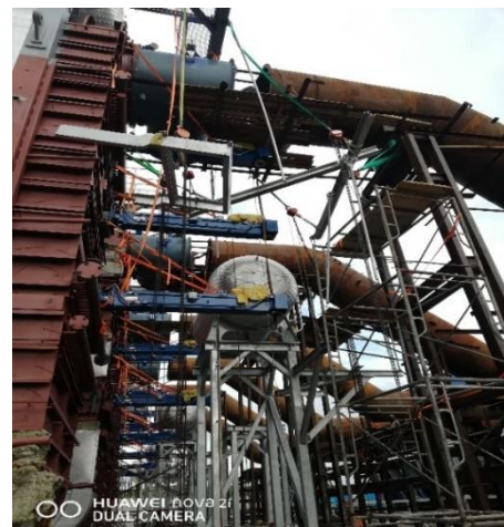
United Ashugonj power Ltd.
